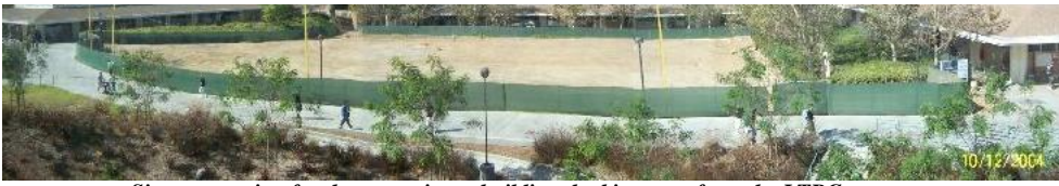
Site preparation for the new science building, looking west from the LTRC
